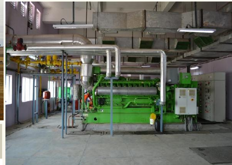
2 MW CBM to power reciprocating facility. Bengal India
